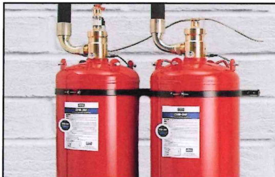
Figure 8: Fire Suppression System
