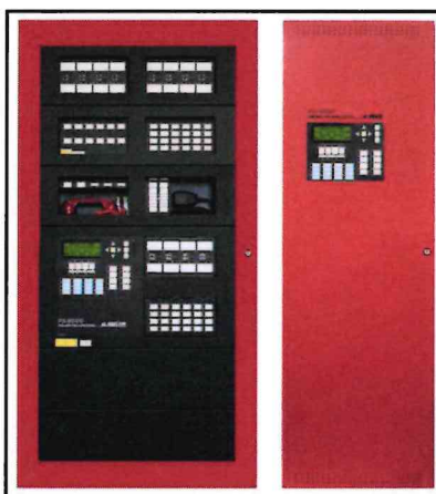
Figure 10: Fire control Panel
